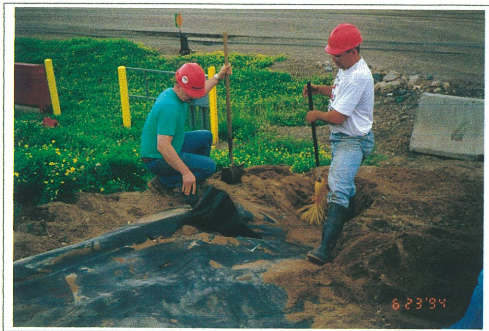
#4 EXPOSING LINER DAMAGE
