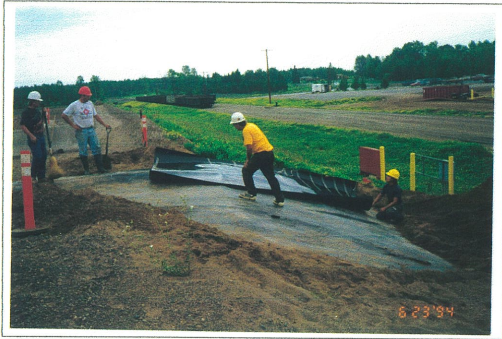
#5 TEMPORARY PATCH OVER AREA MOST DAMAGED
