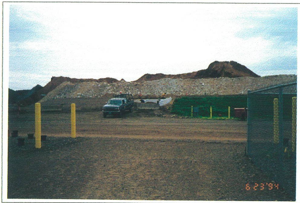
#1 BERM LINER DAMAGE
