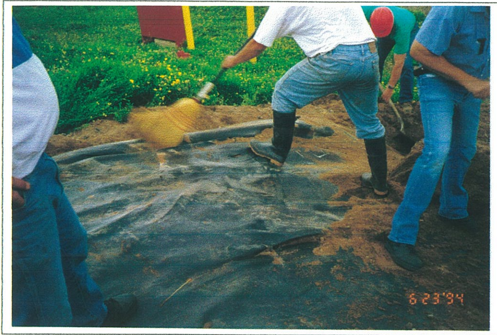
#3 EXPOSING LINER DAMAGE
