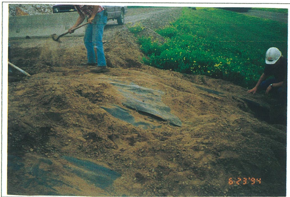
#2 EXPOSING LINER DAMAGE
