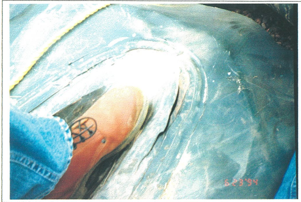
#1 LINER SEPARATION AT DISCHARGE PIPE
