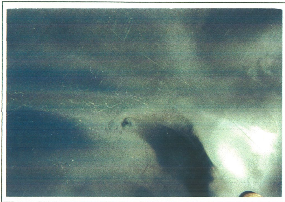
RUNOFF POND HDPE LINER INDENTATION
