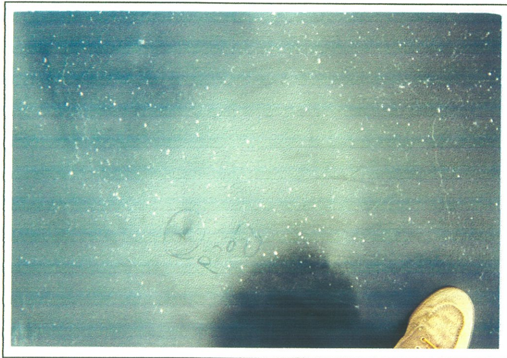
SURGE POND HDPE LINER INDENTATION
