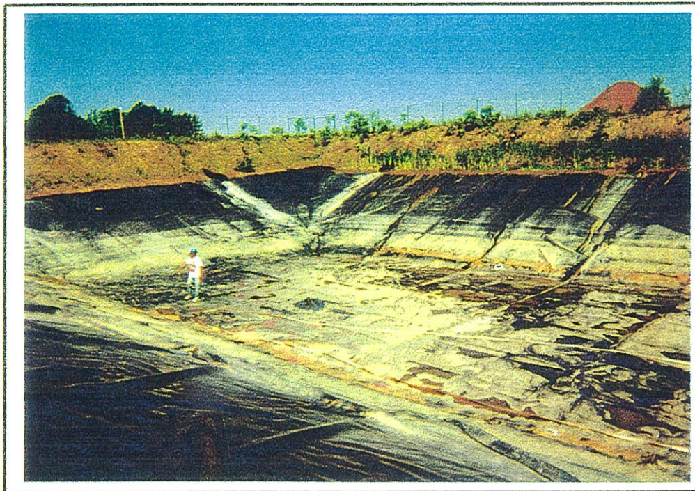
DAMAGE SHOWN IN RED AND WHITE PAINT CAMERA LOOKING WEST
