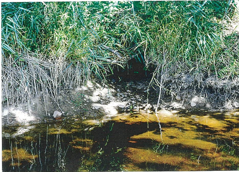
Photograph 5: View of Bank and Erosion Damage Due to Beaver Activity
