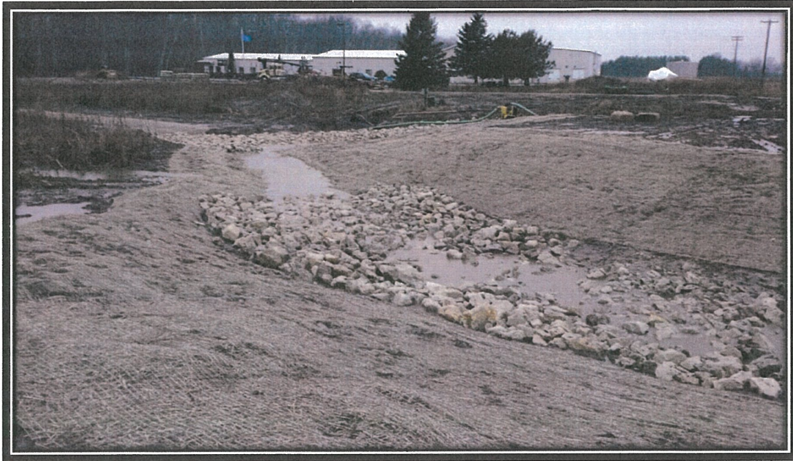
Photograph 20. North and East Area rock-lined swale connection completed and slopes blanketed on November 17, 2015.
