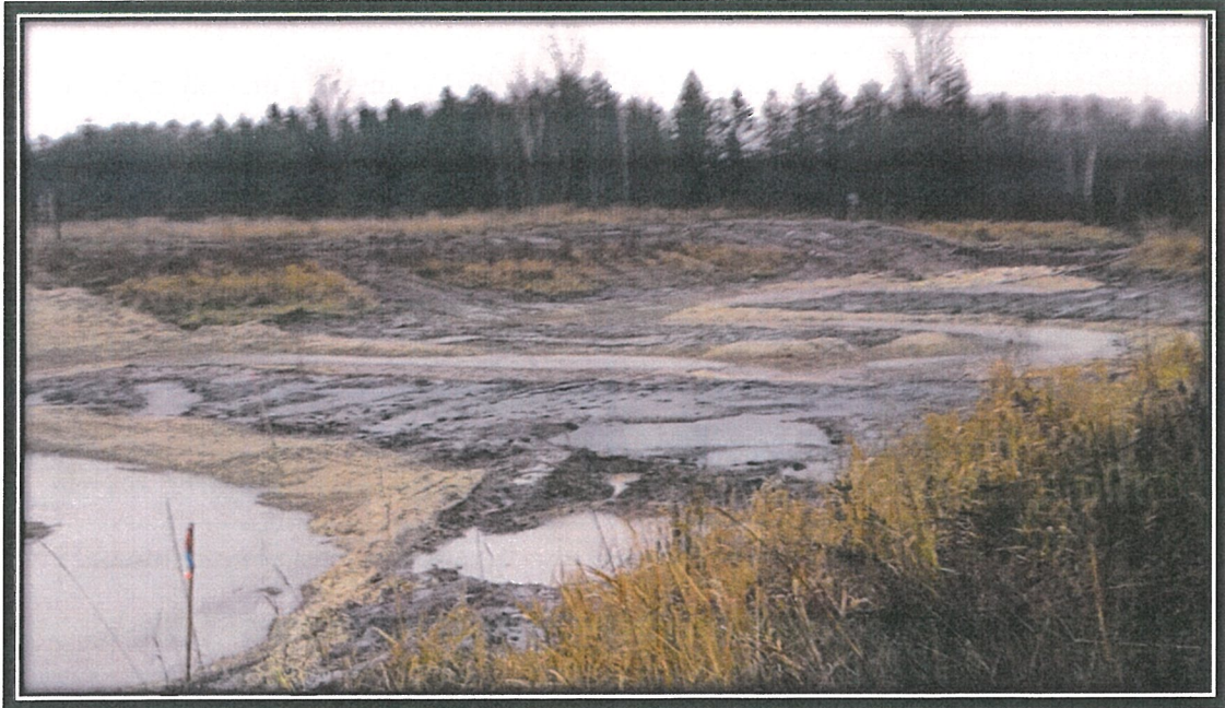
Photograph 10. North Area naturalized low flow channel with erosion blanket installed on November 17, 2015, looking east.
