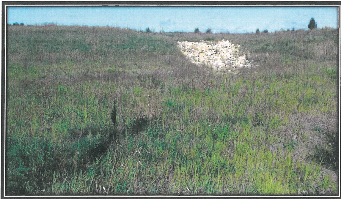
Photograph 18. Surface water inlet in the northwestern corner of North Area, with side slope stabilized on September 8, 2016.
