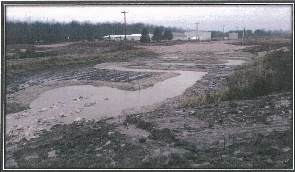
Photograph 14. North Area looking west with naturalized low flow channel erosion control and side slope blanket along western slope on November 17, 2015.
