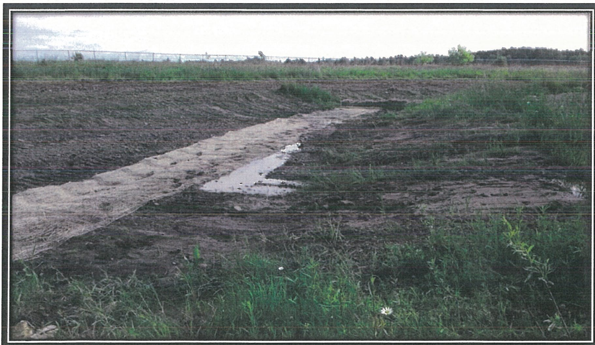
Photograph 22. East-West Swale final shaping and erosion control blanket in place along the swale, June 16, 2016.
