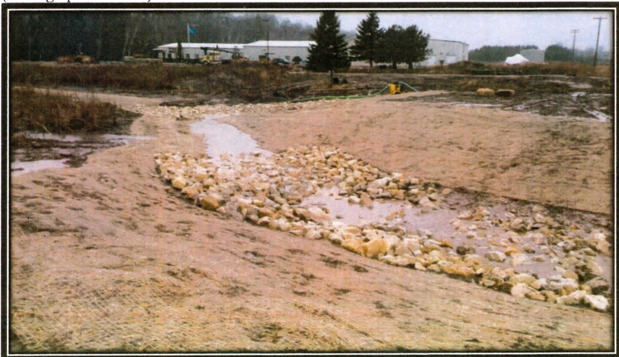
Photograph 25. North and East Area rock-lined swale connection completed and slopes blanketed on November 17, 2015.
