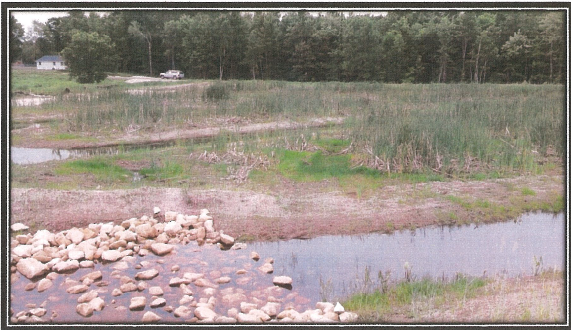
Photograph 6. East Area and naturalized low flow channel with initial seed germination on June 16, 2016. Erosion blanket is still intact.
