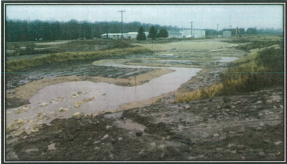
Photograph 17. North Area looking west with naturalized low flow channel erosion control and side slope blanket along western slope on November 17, 2015.
