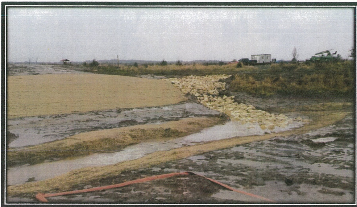
Photograph 21. Surface water inlet in the northwestern corner of North Area with rock rip rap and side slope with erosion blanket in November, 2015.
