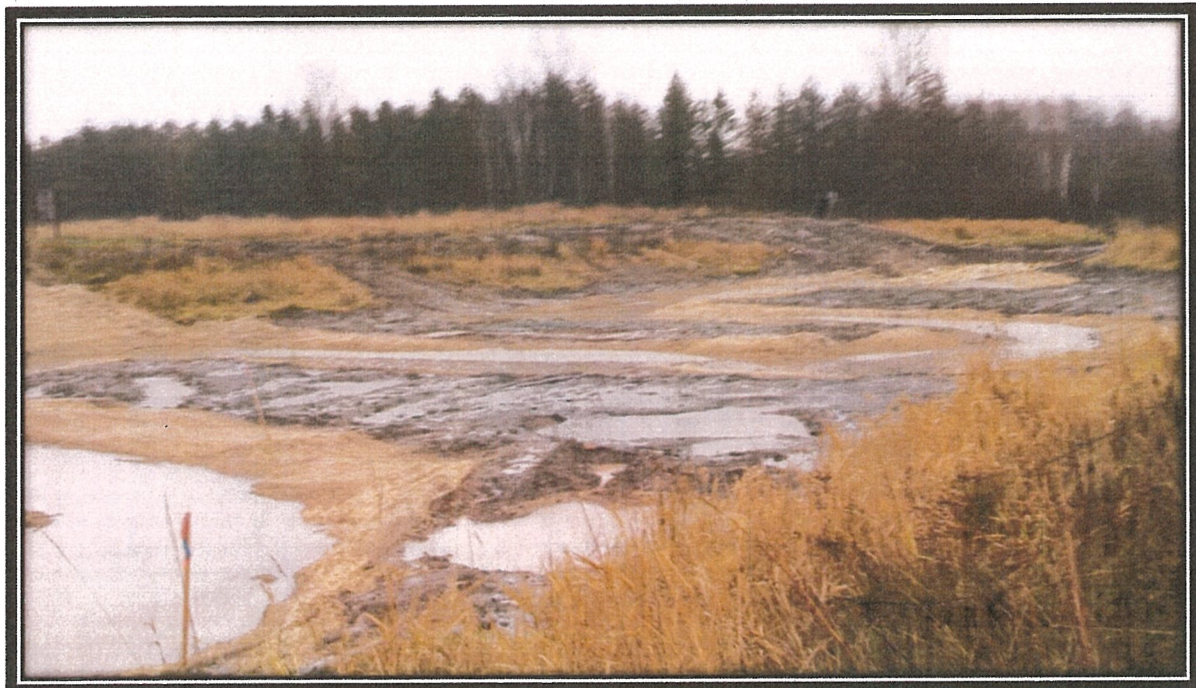
Photograph 12. North Area naturalized low flow channel with erosion blanket installed on November 17, 2015, looking east.
