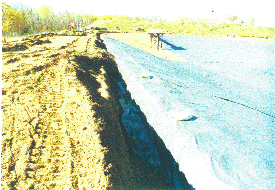
Photograph 7 October 11, 1995 Location: South Pond Description: Partially backfilled anchor trench of south berm.
