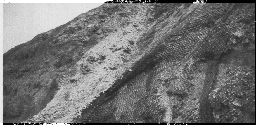
Area where mesh washers failed, allowing accumulated debris to fall onto bench. The majority of such failures occurred where no straps were installed.
