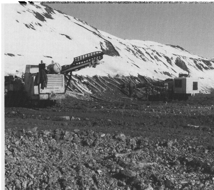
Ingersoll Rand drills were used to install the bolts throughout the pit.
